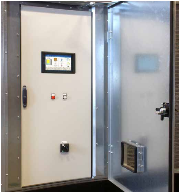
Control cabinet with touch-screen terminal, prepared for connection to the internet.
